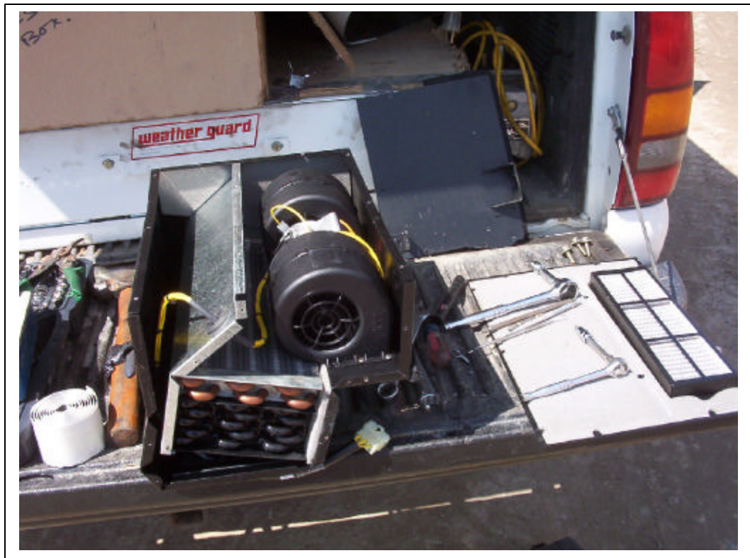
Coils and wiring all back in the box.
